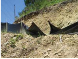
Incorrect Use of Silt Fence
